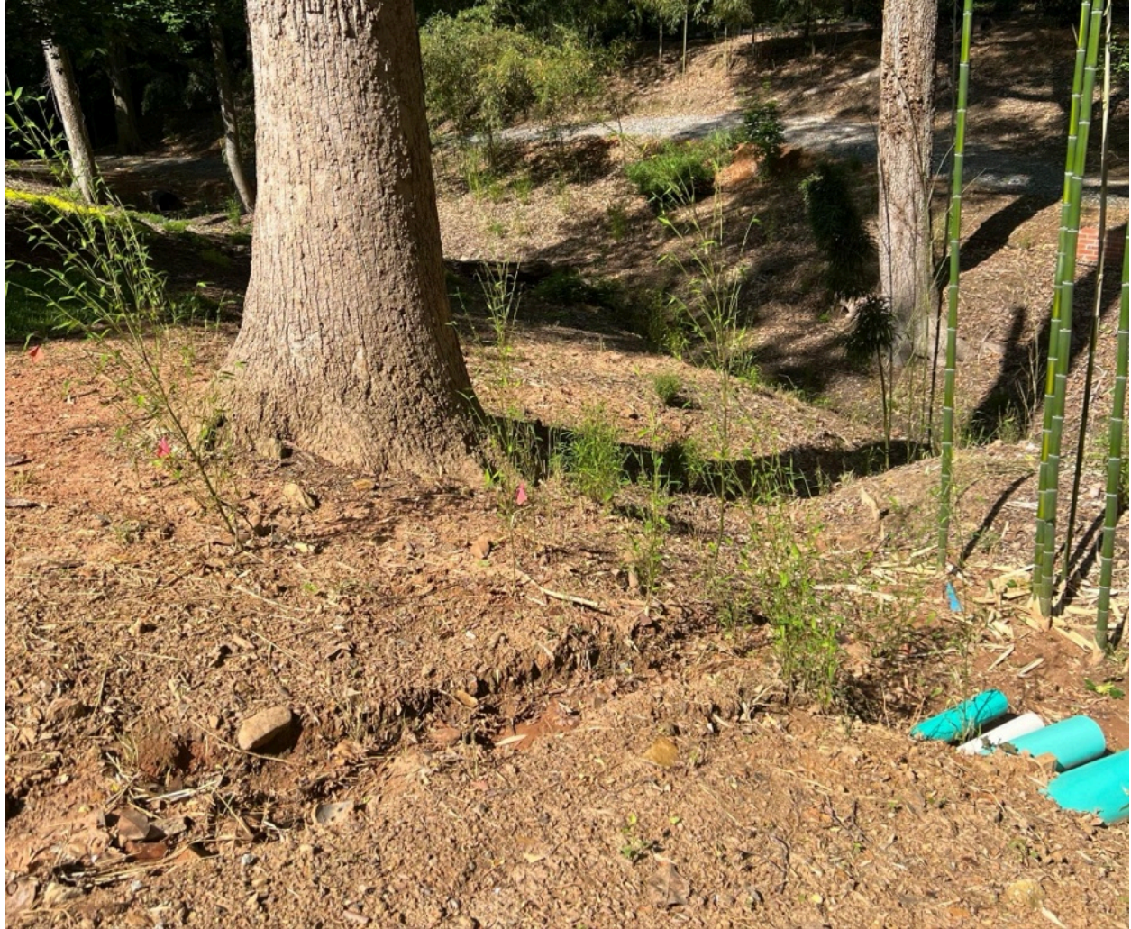
Drainage pipes from house where they spill into the gully at the back of our property.
